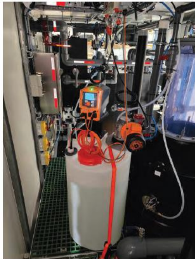
Figure 20: Dosing tank and pump
